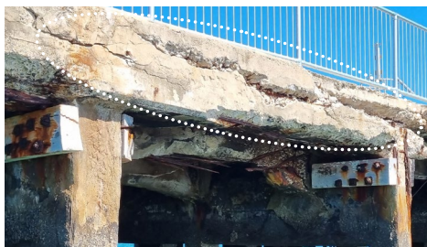
Edge beams: extensive major defects observed.
