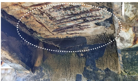
Deck soffit: widespread major defects.
