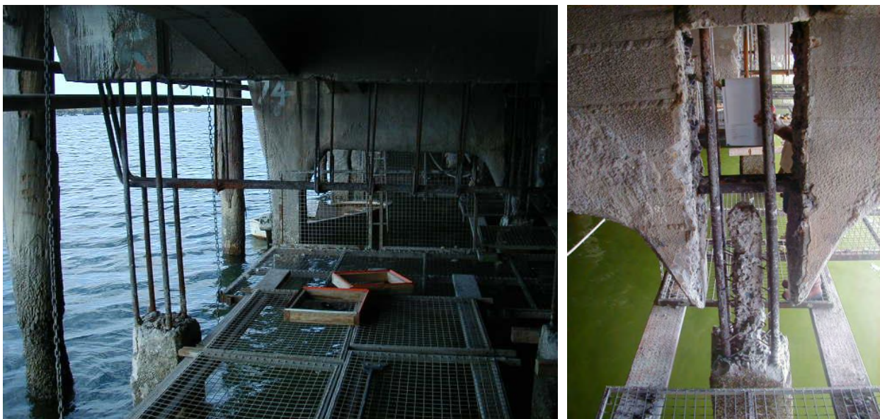
Figure 17: Example headstock and pile below deck repairs with fixed platform system. Note extent of works to be similar to that pictured with full removal and reconstruction of some elements
