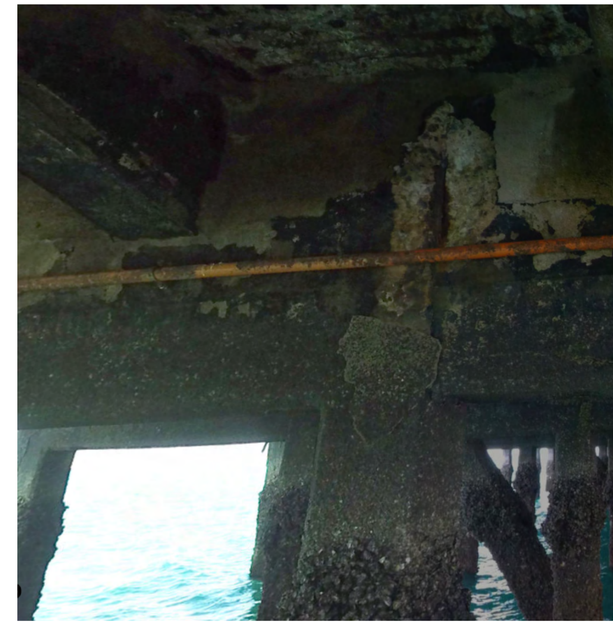
Photo 6 - Pile Spalling at Headstock N.T.S.
