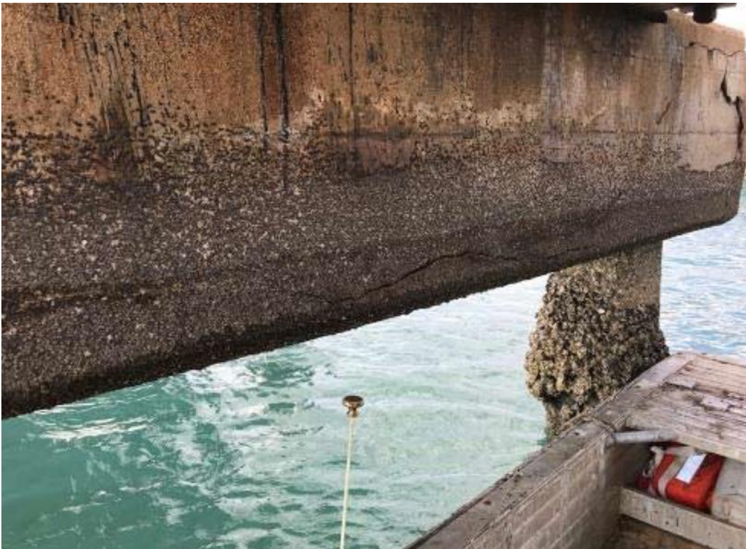
Figure 10: Headstock typical crack close to soffit
