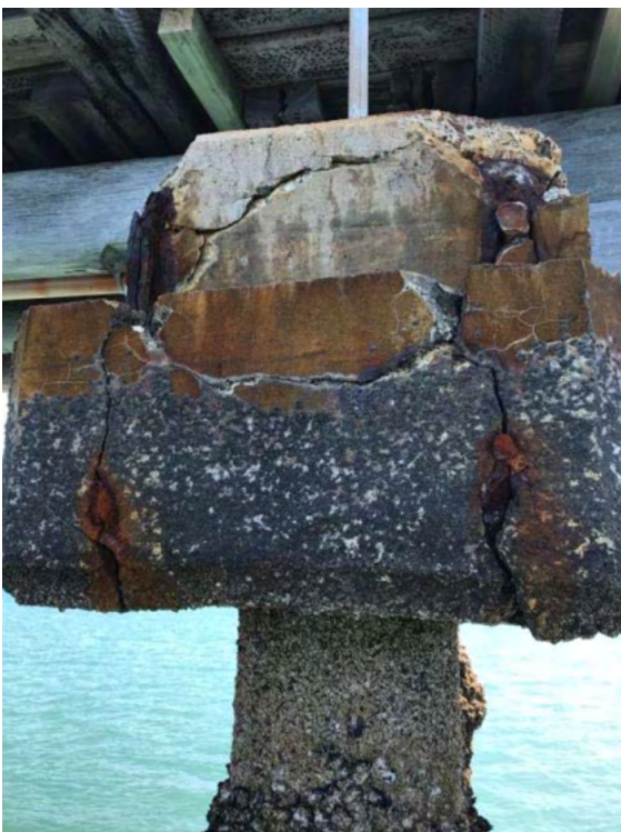
Figure 11: Headstock typical spall at each end
