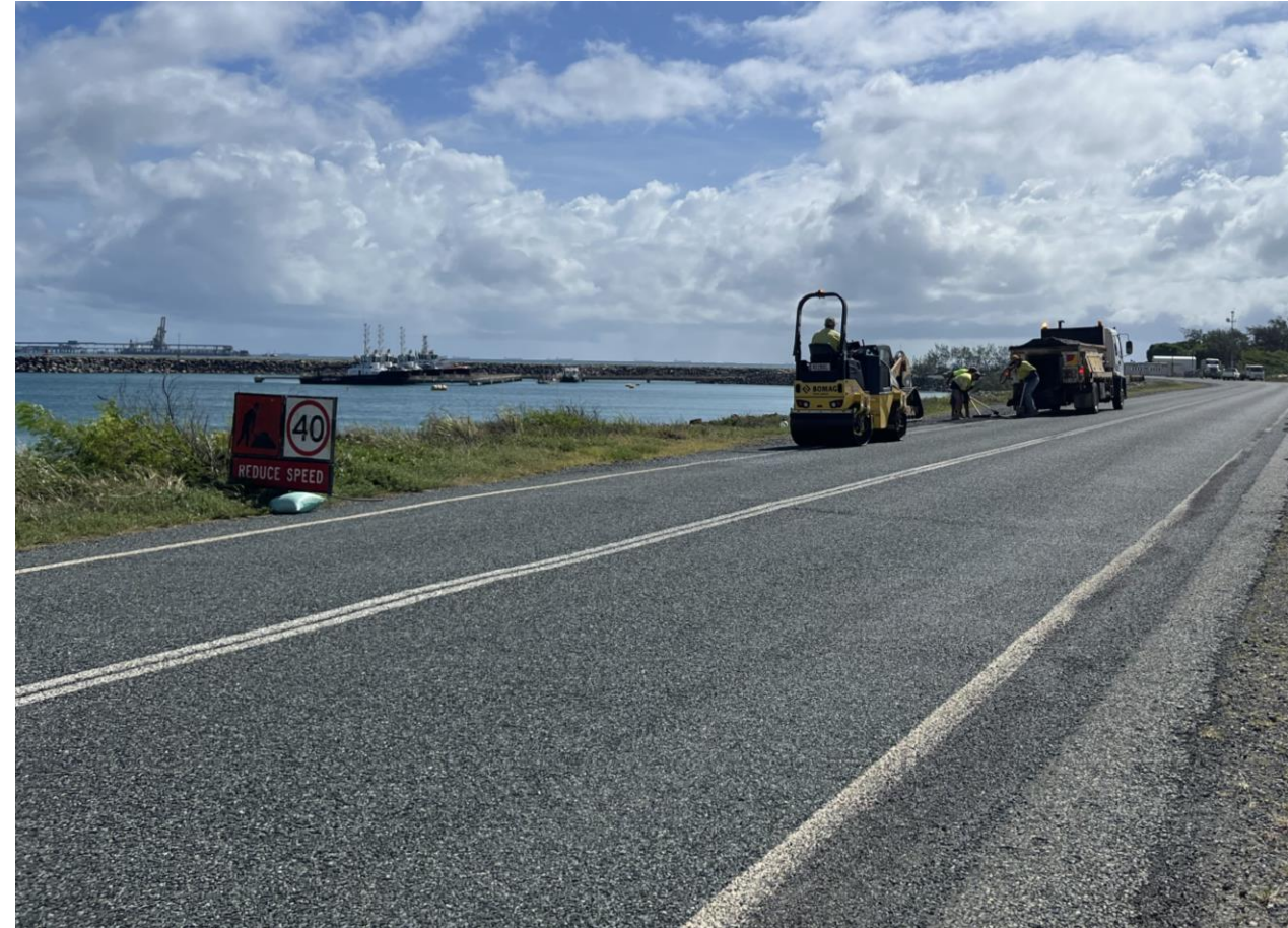
(Above) Completion of edge road works completed at Half Tide Tug Harbour.
