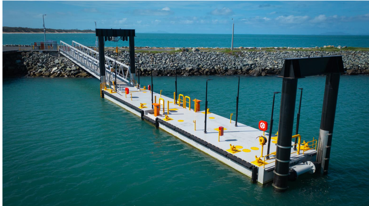
The tug berth gangway and pontoon has been completed on the new tug berth facility project.
