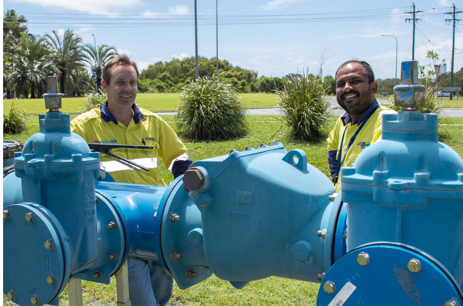
Works on the Water Network Improvement project have been progressing. Pictured: Roebuck Civil Project Manager Craig Bishop & NQBP's Senior Project Engineer Anoop Pillai
