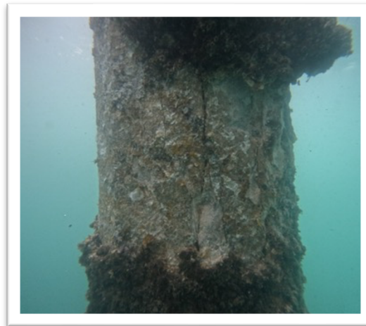
Figure 2: Significant spalling and exposed reinforcement bar towards right edge of upper face 3 (Pile 116D) and face 2 with extensive vertical cracking on upper face 3.
