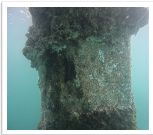
Figure 1: Significant spalling and exposed reinforcement bar towards edge of upper face 2 (Pile 116D) and face 3 with significant material loss.
