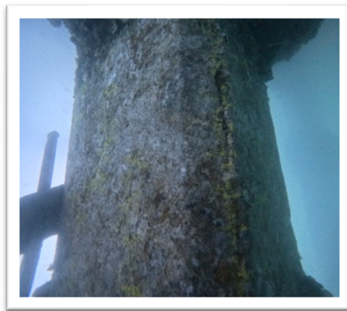
Figure 3: Large vertical cracking at edge of upper face 3 and 4 with crack width to 20mm and rust staining towards lower end of crack.
