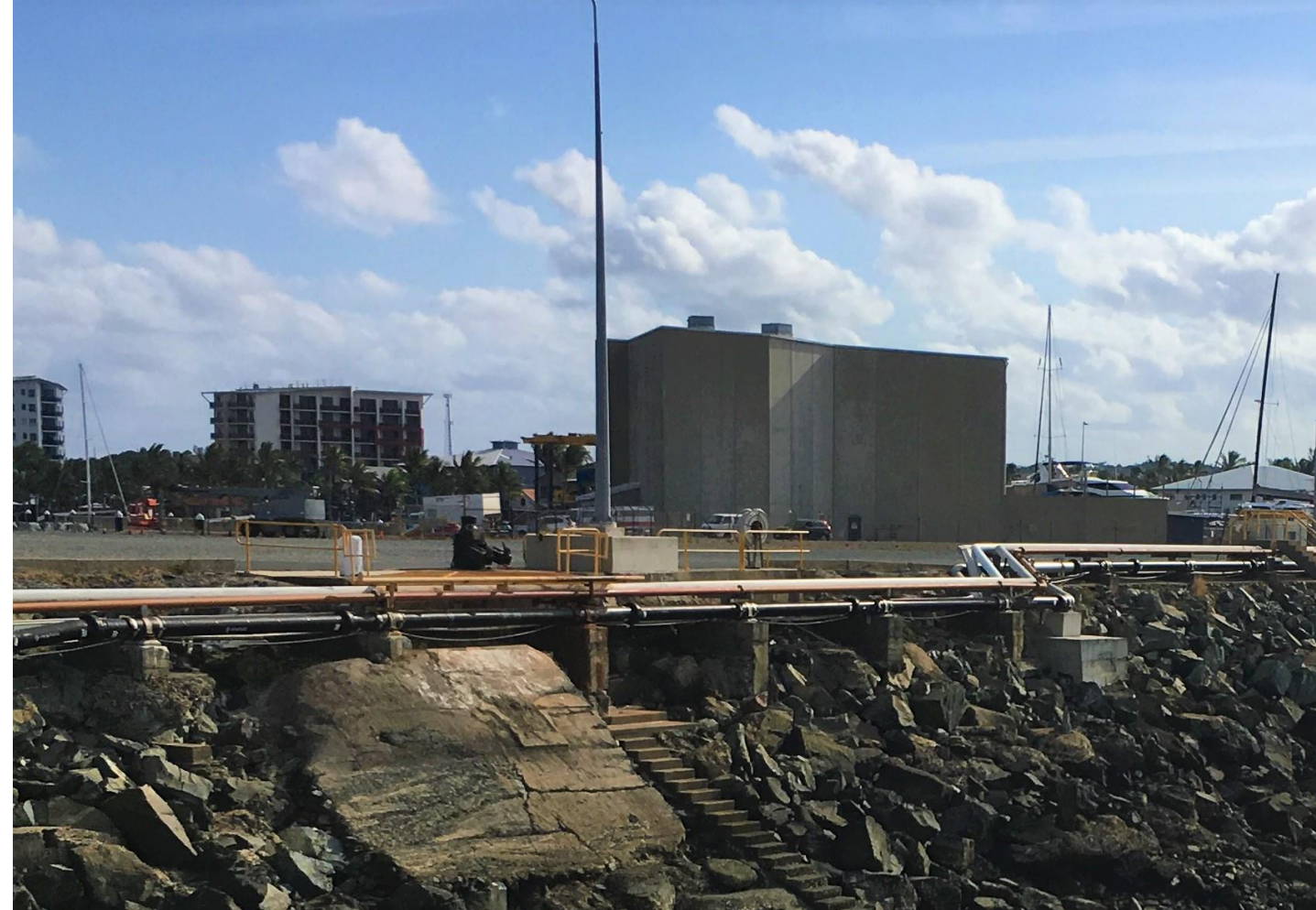
Fuel pipelines at Wharf One.
