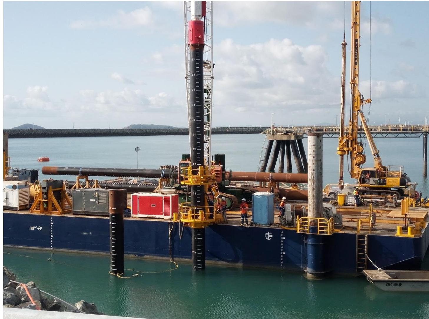
Pile driving works were recently completed on the new tug berth facility project.
