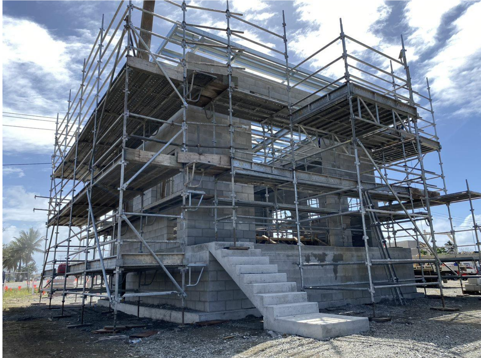
Pictured: Fergus Builders are progressing construction of the new water booster pump station on Harbour Road.
